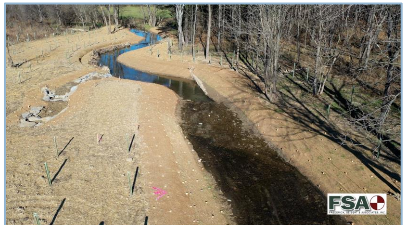
The project resulted in a total of 2,700 linear feet of uninterrupted stream that is now reconnected to the floodplain.
